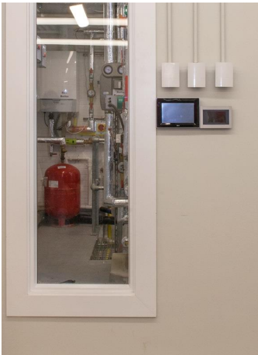
A look into the Plant room and the CHP system located in every room.
